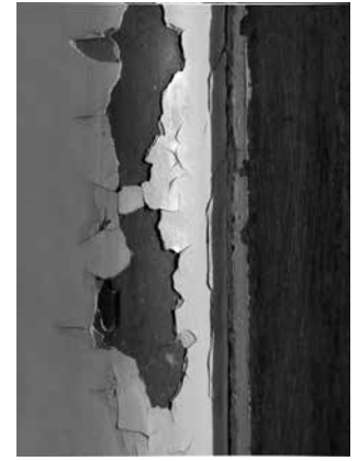
JOSEF FRANK AND OSKAR WLACH, VILLA BEER IN VIENNA-HIETZING, 1930, WEST FACADE, MAIN ENTRANCE, METAL DOOR FRAME, DETAIL WITH REMAINS OF THE ORIGINAL "JAPANESE RED" PAINT
